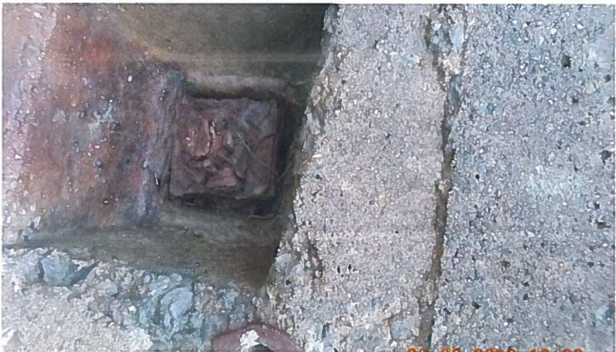
Lateral Tension Rod - Rust with Section Loss (Typical)
