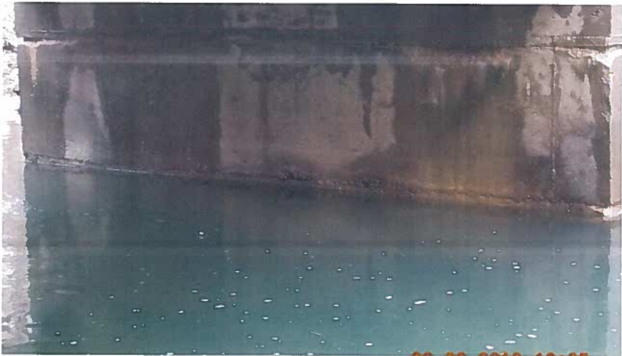
Abutment 2 Elevation - Minor Vertical Cracking, Spalls along Construction Joint and Staining from Leaking Joints
