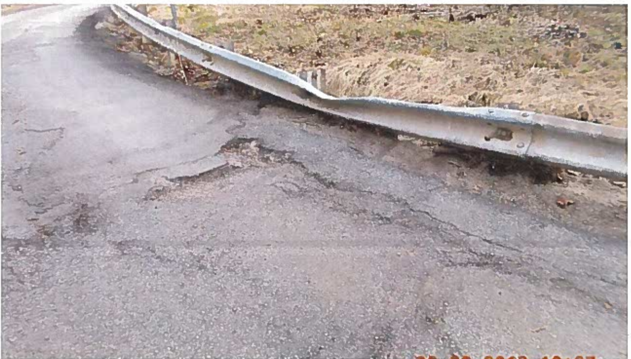
Guardrail Damage at Northeast Quadrant
