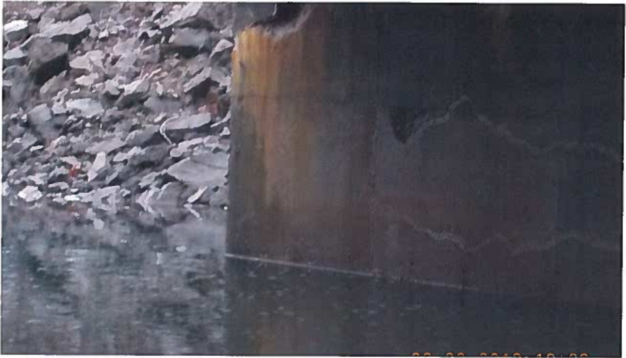
Abutment 1 Spall and Cracking on East Side
