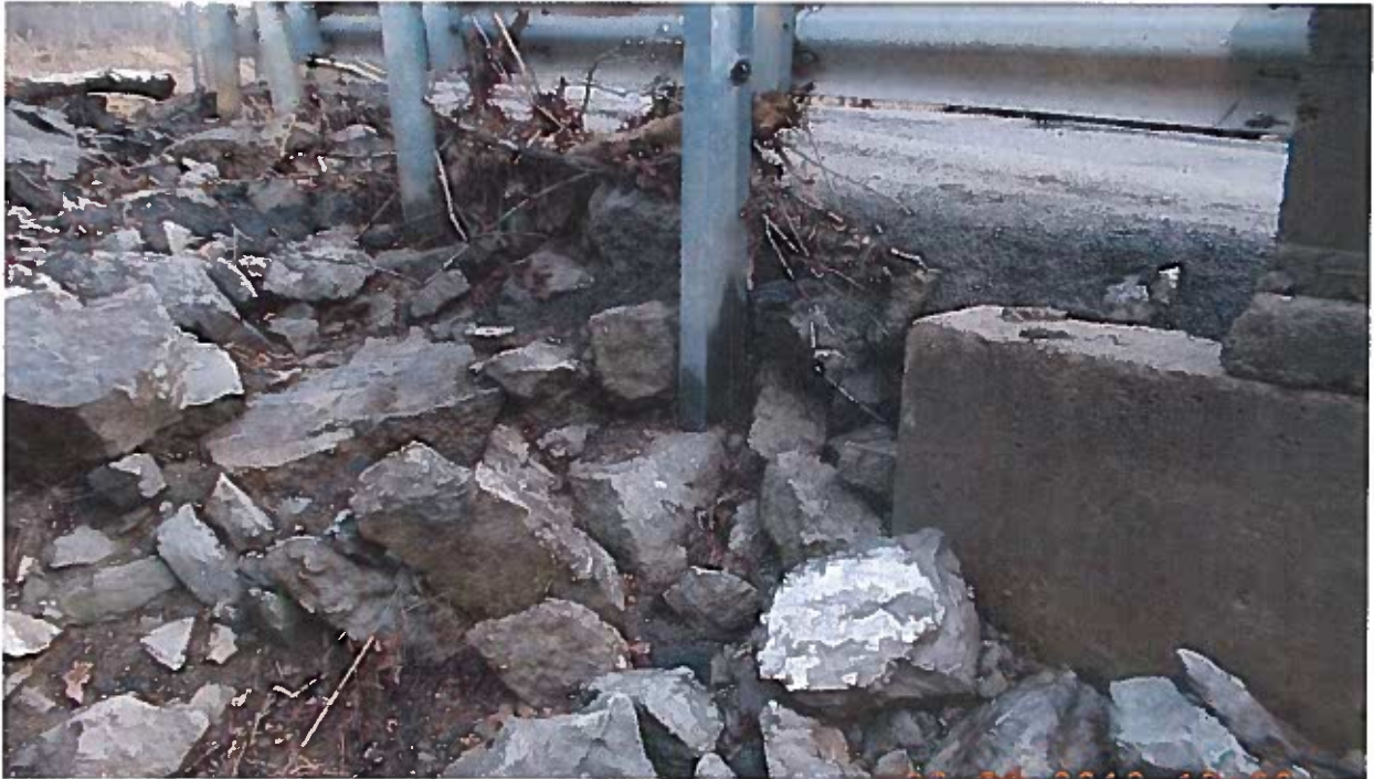
Guardrail Post not Embedded - Erosion and loss of Fill at Northwest Quadrant
