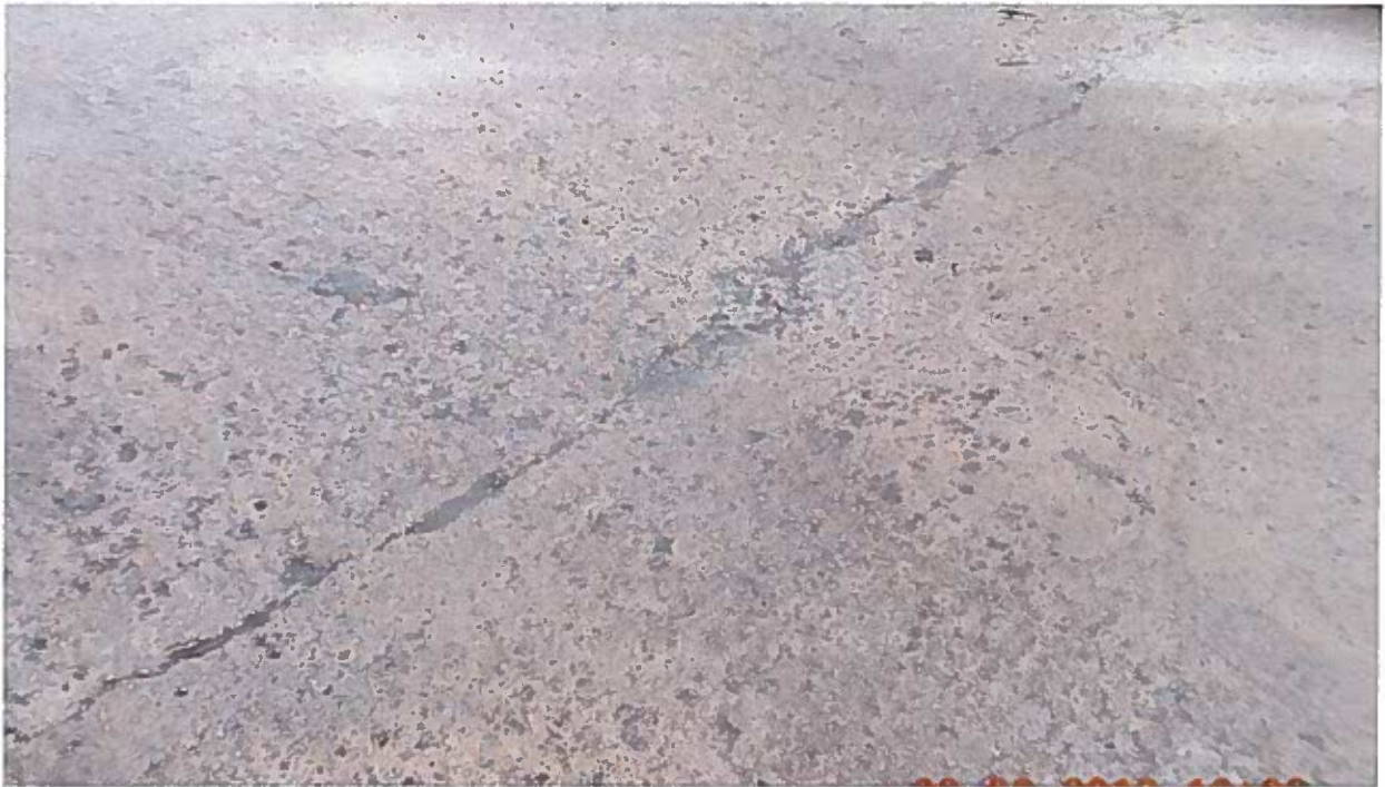
Transverse Cracking in Approach Slab - Typical
