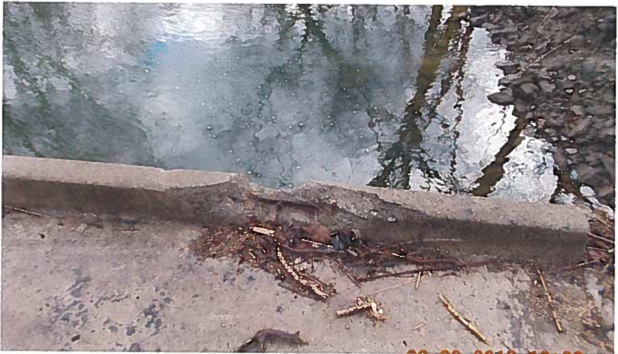
East Curb Spalled with Exposed Reinforcing Steel
