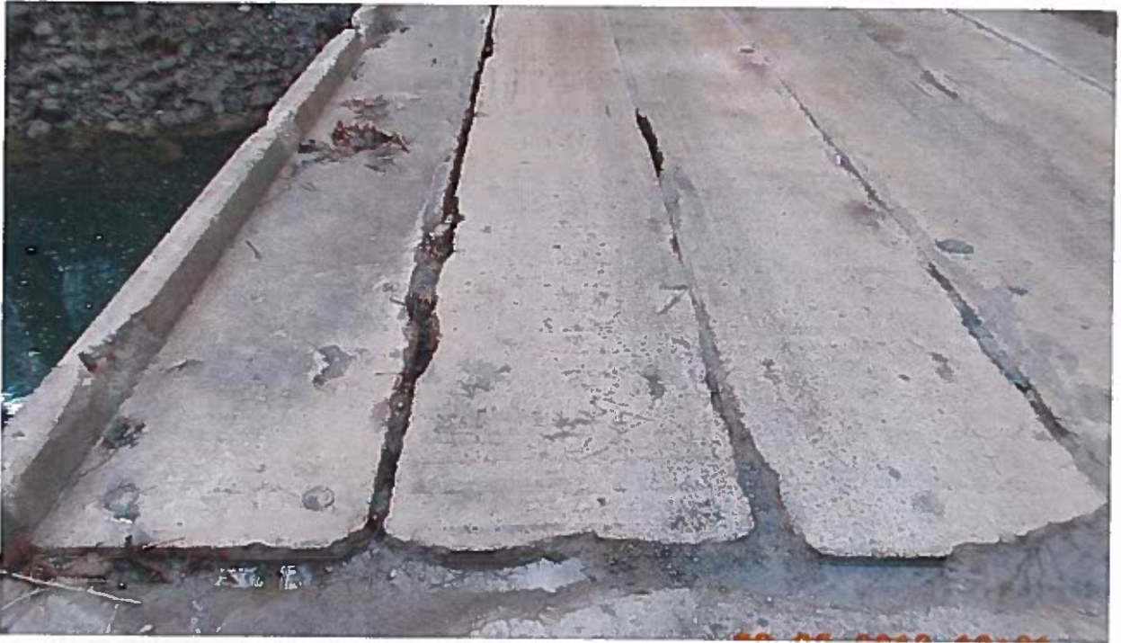
Deterioration of Joints between Beams - Looking South
